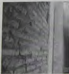
Fig. 303. S. Sustina. South wall of nave, (restored), double window, blocking in false column.
